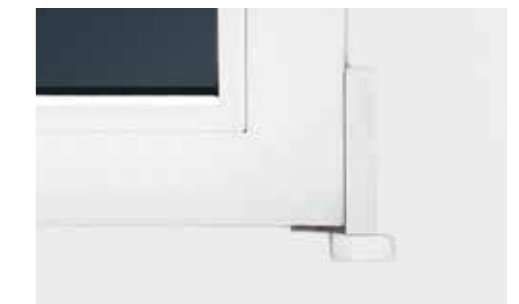
Exposed hardware parts
